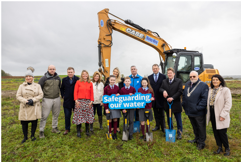
Cathaoirleach Cllr. Nick Killian pictured at the official sod turning of The Windmill Hill Reservoir and Trunk Watermain to Ratoath project
