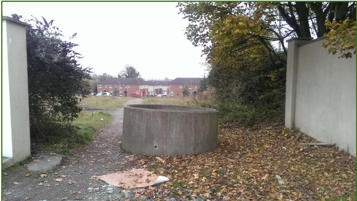
The drainage pipe at the entrance to the vacant site in Longwood
