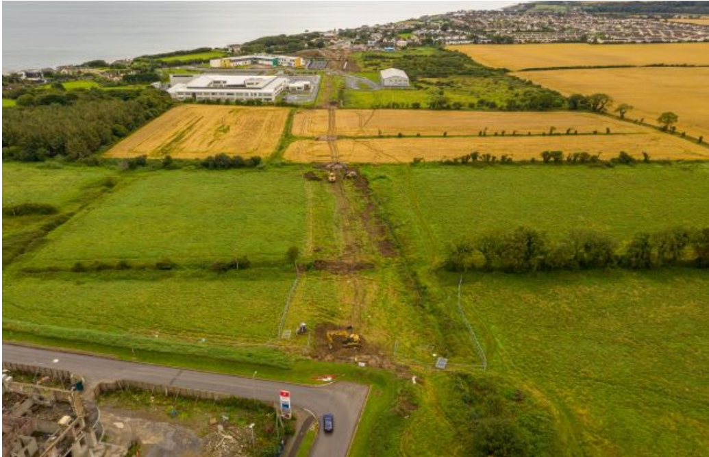
Work commenced on the R150 Laytown to Bettystown Spine Road in early August
