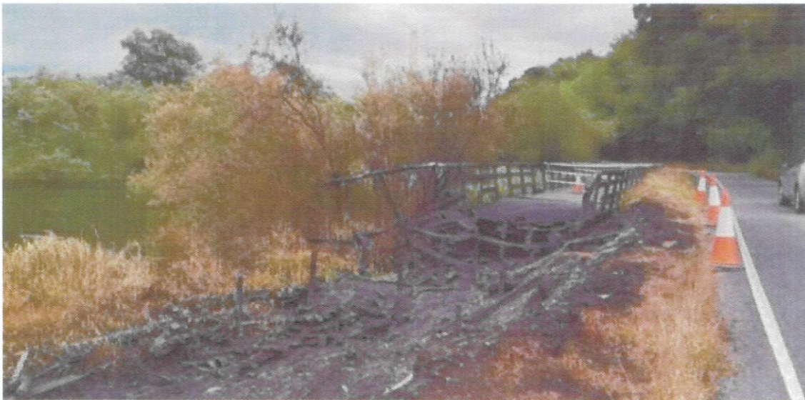
Portion off the fire damaged Boyneside Trail pathway. 26 th July, 2018
