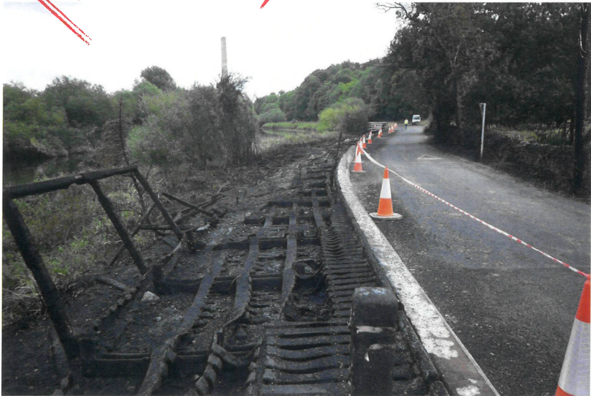
(Result of arson damage to Boyne Greenway near Oldbridge on 26 July 2018)
