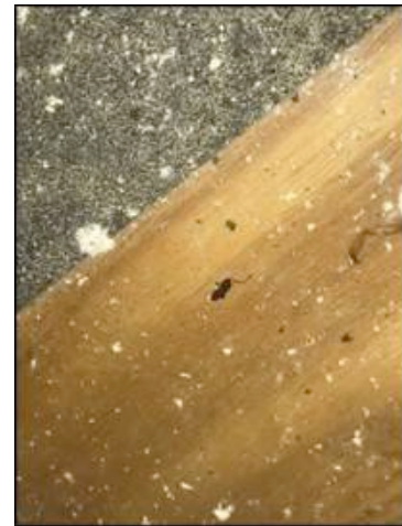
Figure 8: Photograph of bat droppings on the staircase of the bell tower
