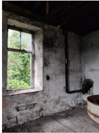
02: Building is currently open to the elements. Existing timber windows in poor repair.
