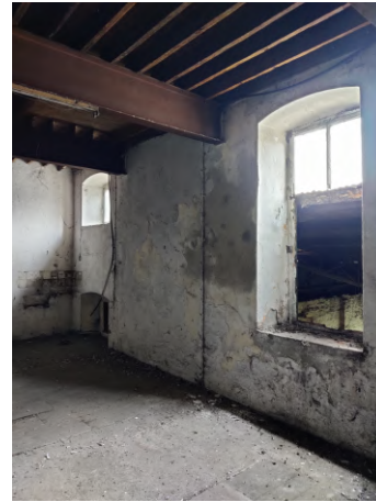
03: Steel and timber floor joists exposed to underside of second floor. Original windows to corner indicate original floor levels when 4 storey Corn Store existed.
