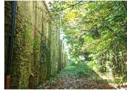
04: Rear of building, original 'patchwork quilt' of masonry records the history of the site's development.
