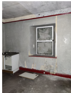
11: Infilled windows to eastern GF room. R.0.B2
