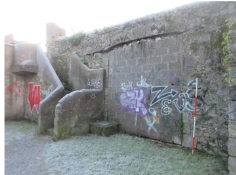
Step Access [24] and Blocked Gate [25]
