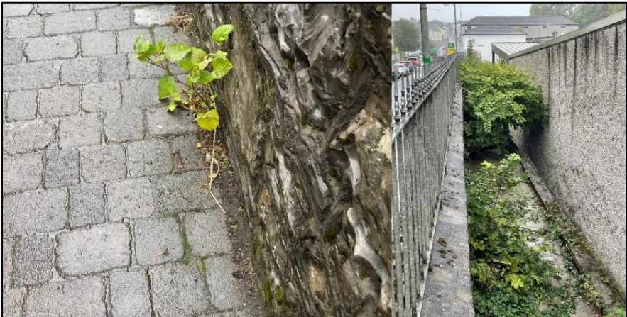
Figure 34: Population of Japanese Knotweed undermining wall at fore of buildings
