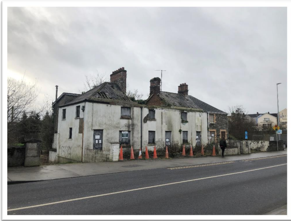
4 no. Derelict Terraced Dwellings
