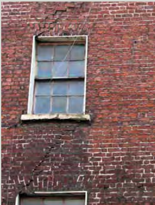
Façade brickwork showing evidence of structural movement in the cracks stretching between the windows
