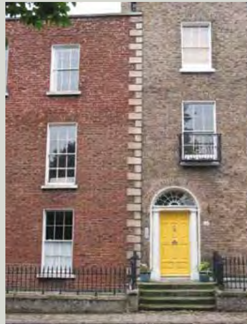
Colour-washed façade brickwork can be seen to the building on the left
