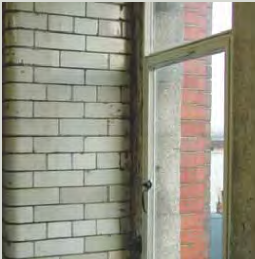
Glazed bricks, in white or pale colours, were often used to the sides of windows and in light wells to reflect more light into the interior of a building
