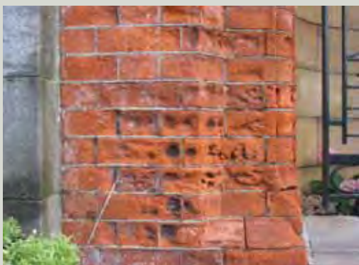
Weathering of brickwork can in some cases be severe. In this case, the decay may have been exacerbated by the mortar being too strong
