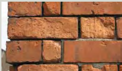
The mortar has weathered back or been washed out of this brickwork to a severe extent and it is now in urgent need of repair and repointing
