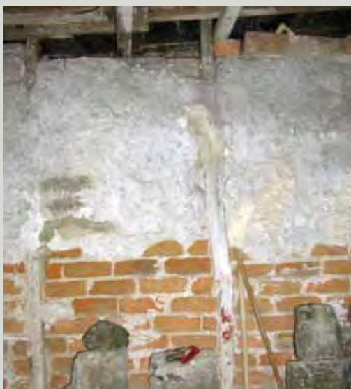
Handmade brick used in a brick nogged internal partition, now exposed where the original plaster coating has fallen away
