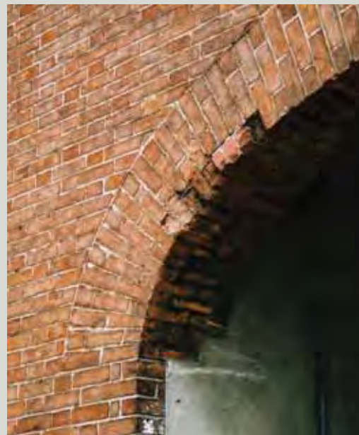
Bricks can be damaged by impact, in this case from a vehicle striking a brick archway
