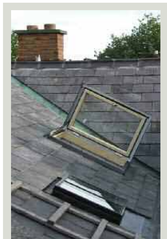
This modern double-glazed skylight allows access to a concealed valley gutter for maintenance inspections and cannot be seen from ground level. It also lets additional natural light into the attic space below
