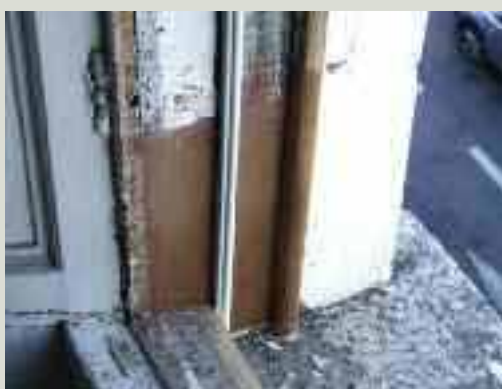
A repaired window frame with a replaced style and new parting bead. The timber sash frames have been temporarily removed
