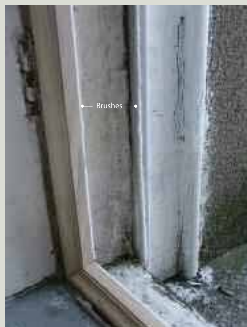
Draught-proofed window frame: brushes are visible on the staff and parting beads, both of which have had to be replaced in order to draught proof. For the brushes to work properly it is important that they are not painted over
