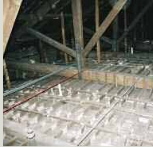
A large roof space with no insulation above the ceiling; while the heat rising from the building interior may benefit the timber and other building materials in the roof space, a lot of energy is wasted in this way
