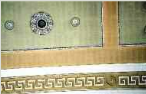
This plastered ceiling has no insulation above it. Discolouration can be seen on the plasterwork between the timber joists located above, as the timber is slower to transfer heat to the cold roof space than the plaster alone. Dust particles in the warm air passing through the plaster remain trapped on the surface causing the discolouration
