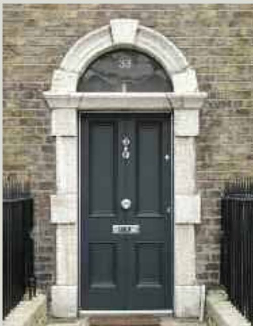
Aluminium draught strips can be seen to all sides of this door. The metal part of these strips, unfortunately visible, can be painted (although it is difficult to achieve successfully) but it is important that the flexible sealant strip is not
