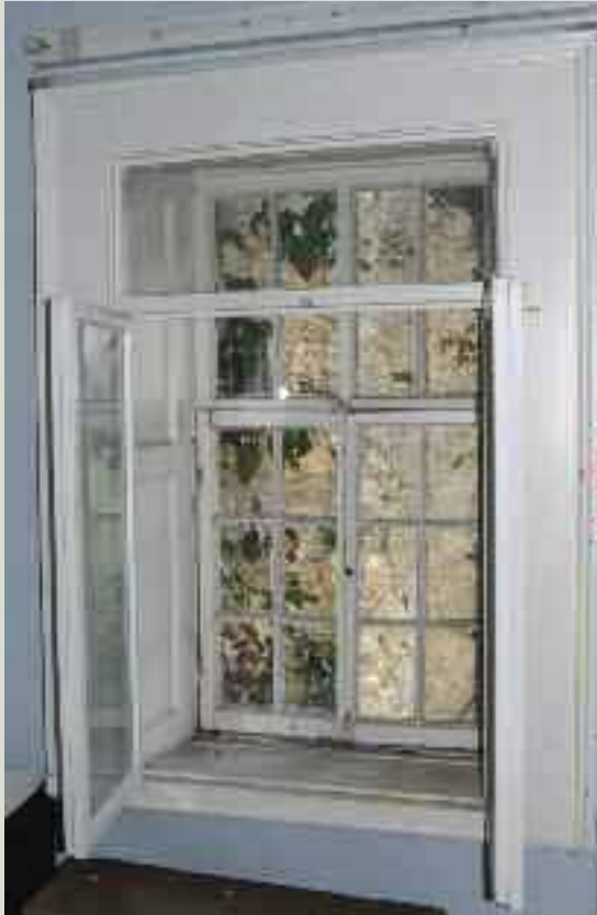
An Edwardian window with 1950s secondary glazing. The secondary glazing is chunky and does not match the original window profile and blocks light from the room. The position of the frame within the opening prevents the shutters from being used
