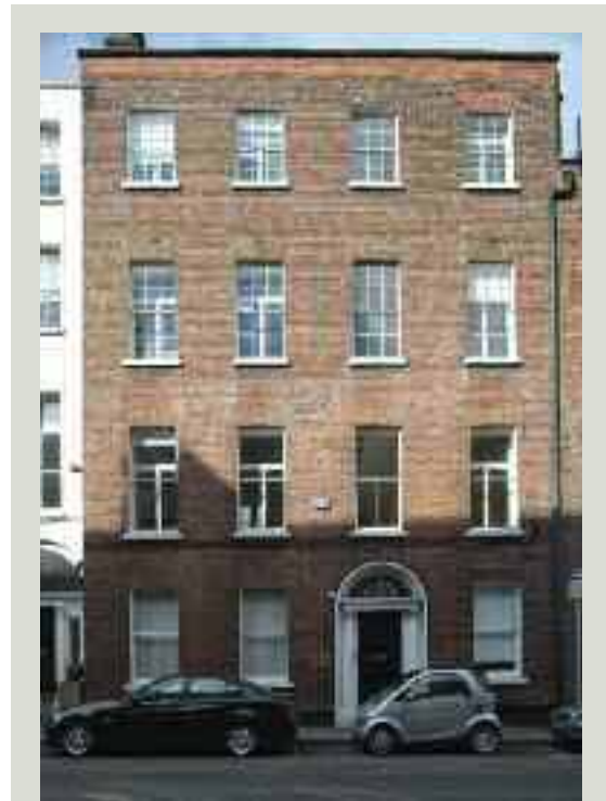
Inappropriate timber-framed secondary glazing with frame proportions that do not match those of the original window, creating a discordant appearance
