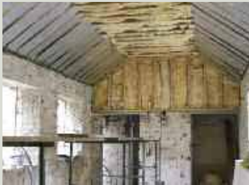
As part of the complete refurbishment of this building, the opportunity was taken to insulate the roof. Rigid insulation has been fitted between the rafters in the sloping sides with quilted insulation fitted between the ceiling joists across the top
