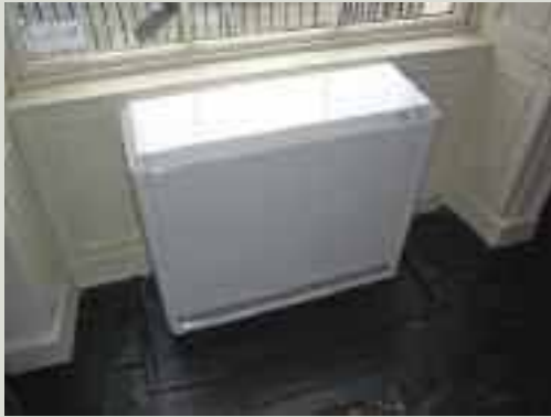
A storage heater fitted in a Georgian house. The low height of the storage heater allows for operation of the shutters at night and does not block the window
