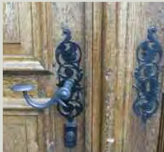
Often the original door furniture is finely crafted to provide ease of use. In this case the lever door handle can be used with minimal effort
