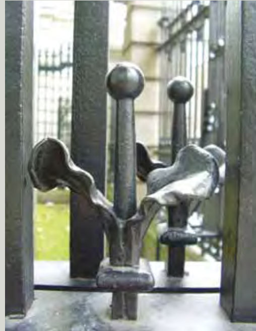
A new section of gate, based on the design of the adjacent gate at the entrance to Leinster House, Dublin. To prevent corrosion, water traps should be filled so that they shed water, or pinholes drilled at the base to allow water to escape (although drilling into original fabric should be avoided where possible)
