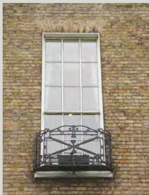
Due to their position and the potential for injuring people below, balconies and balconettes should be periodically inspected to ensure that they are secure
