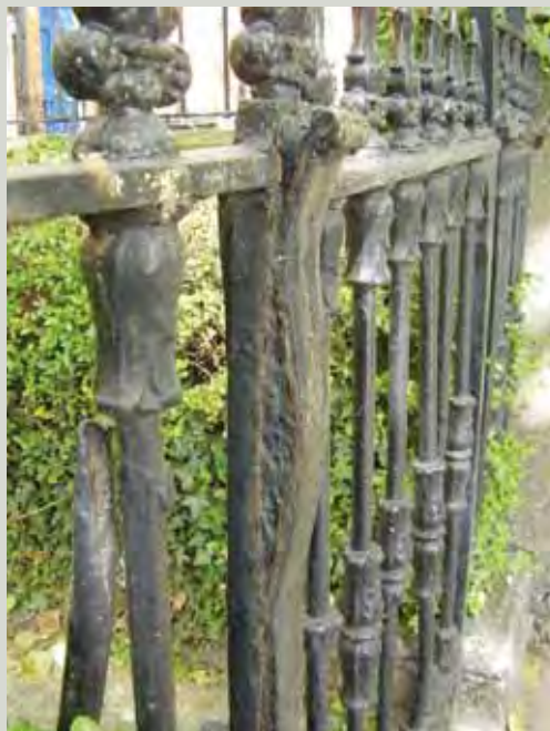
Corrosion between the gate frame and slam bar is common
