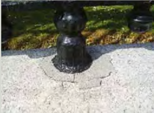
Crushed stone mixed with mortar has been used to fix this ironwork into the masonry socket
