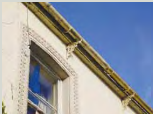
Cast iron gutter brackets, typical of the second half of the nineteenth century
