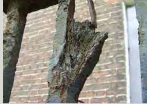
Wrought iron typically 'delaminates' as it corrodes, accentuating the fibrous structure of the material
