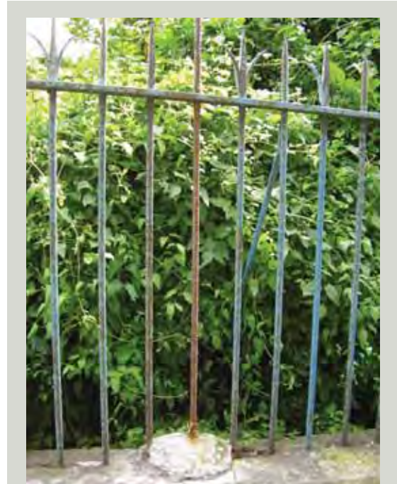
Repairs should be sympathetic to the design and traditional detailing of ironwork unlike this repair which is damaging to the appearance of the railings, will damage the stone coping and is likely to fail
