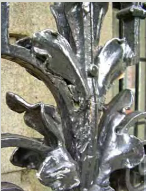
Water traps, such as the void areas behind these leaf details, will cause corrosion to develop at a faster rate
