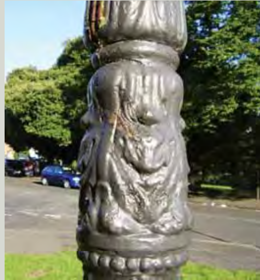
Over-thick application of paint will obscure detail and result in less effective protection
