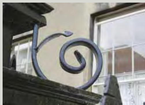
It is important to choose an experienced craftsman to avoid inappropriate repairs. The replacement scroll in the lower image has been crudely formed and bears little resemblance to the finely-crafted original feature on a neighbouring property in the top image
