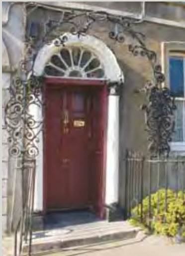
This is a rare example of superb late eighteenth-century wrought ironwork. This highly ornate arch required considerable skill to make
