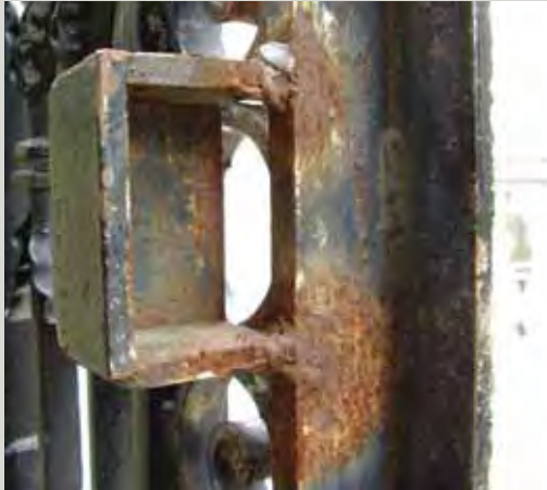
Galvanic corrosion is occurring between the original wrought iron gate frame and the metal of the filler rod that was used to form the weld joint attaching the gate catch to the gate frame
