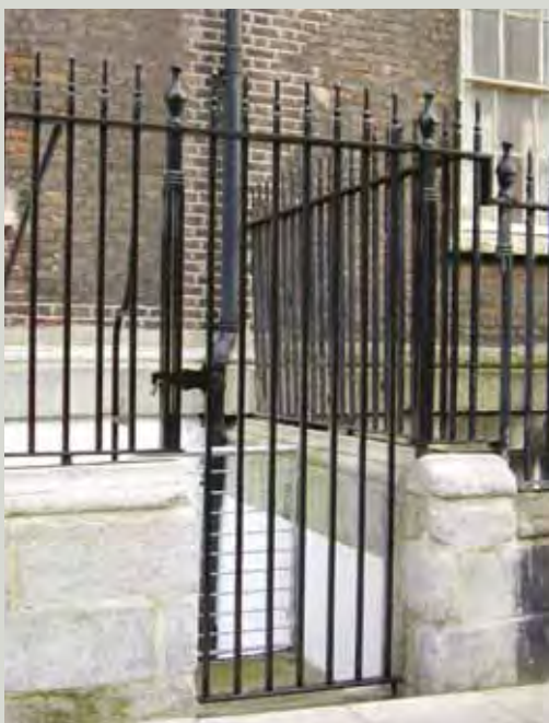
This replacement gate has been inserted sensitively and has been designed to tie in with the proportions and design of the original railings
