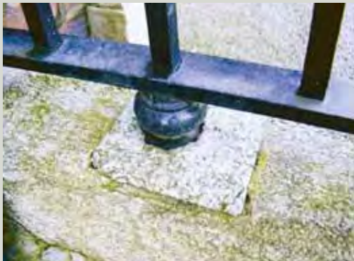
A stone indent has been inserted to repair a fracture or widened socket
