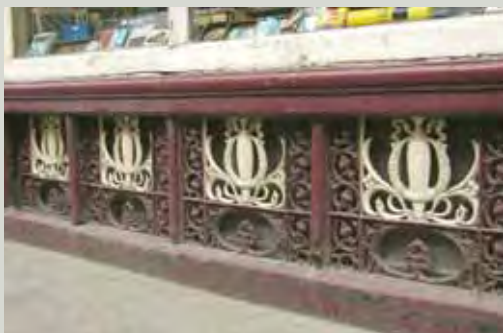
Routine maintenance to ironwork, such as this attractive cast iron stall riser to a shopfront should include gentle washing using a minimum amount of water to remove accumulated dirt
