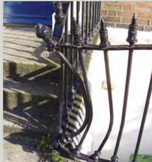
Impact damage caused for example by vandalism or cars, can cause deformation (in the case of wrought iron) and fracturing or shattering (in the case of cast iron)
