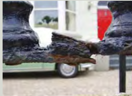
Corrosion developing at a scarf joint
