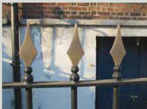
The original cast iron finial is depicted on top. Mild steel replacement finials are shown below. These are flat and poorly designed in comparison to the original and have been individually welded onto the rail
