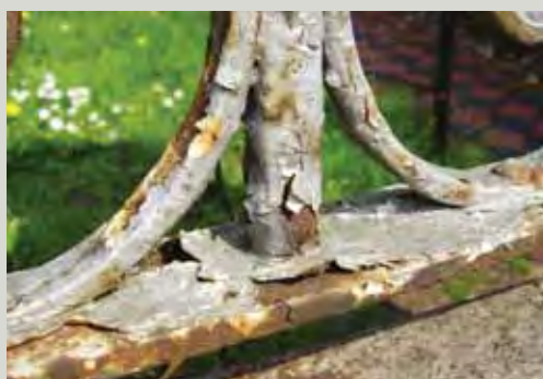
Broken, flaking paint traps and holds water to the iron, preventing it from drying out properly, and can lead to corrosion. Areas of chipped paint are not as significant a threat so long as the iron is in an exposed location and is able to dry out. Nevertheless, such chips should be treated as soon as possible to prevent rust from forming
