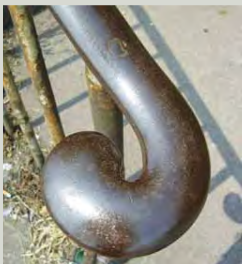
An oxide layer has developed on this wrought iron handrail which protects it from further corrosion
