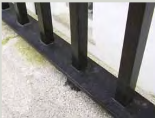
Replacement bars should pierce through the rail rather than be welded to it (as shown above)
