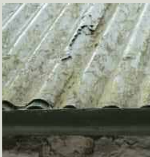
Crevice corrosion is frequently a problem with corrugated iron, particularly at the laps between corrugated sheets
