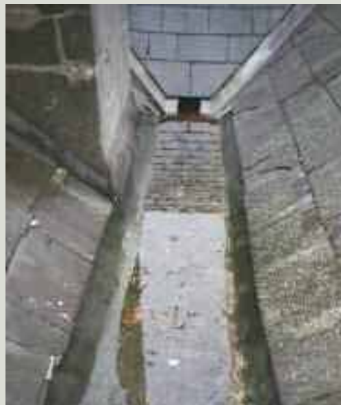
View of a defective valley gutter with a shallow fall that is now holding water. Birds' nests in the outfall of the secret gutter (seen at the top of the image) blocked this roof outlet
