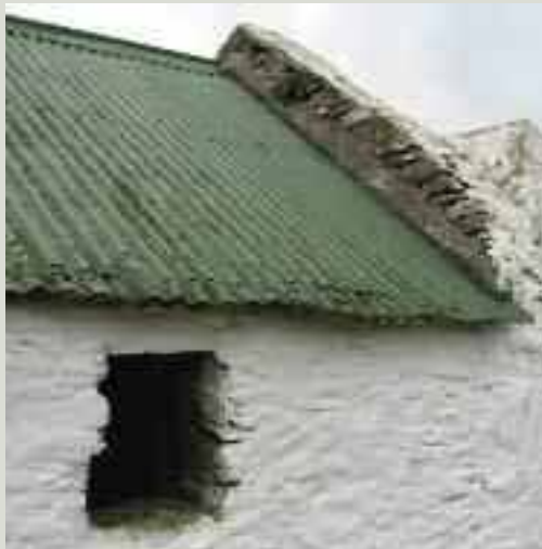
The eaves edge of corrugated-iron sheeting is particularly vulnerable to corrosion. Here, additional layers have been inserted under the eaves
