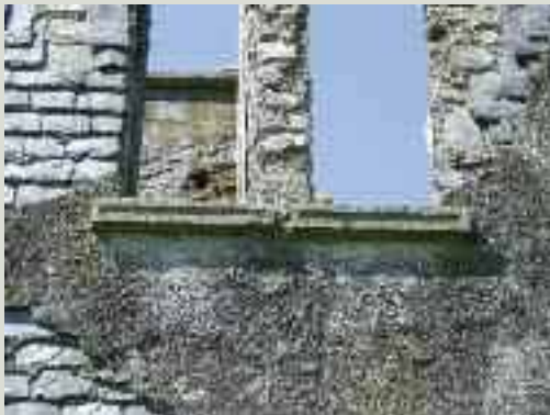
On this ruinous house in County Cork, the vertically hung slates, bedded in lime mortar, were later rendered over. Their existence only came to light as the external render decayed and fell off
