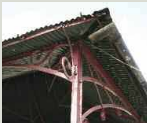
This corrugated iron is suffering from pitting, visible as small pinpricks of light where the metal has corroded through. There is also crevice corrosion occurring at the junction of the sheet with the hip roll. In addition, work is urgently needed to repair the rainwater goods
