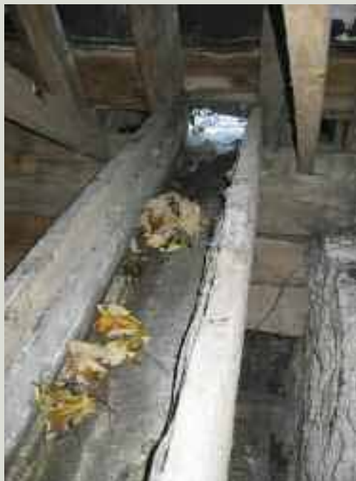
A lead-lined, secret gutter within the roof space used to carry rainwater from an internal roof to outfall at the eaves
