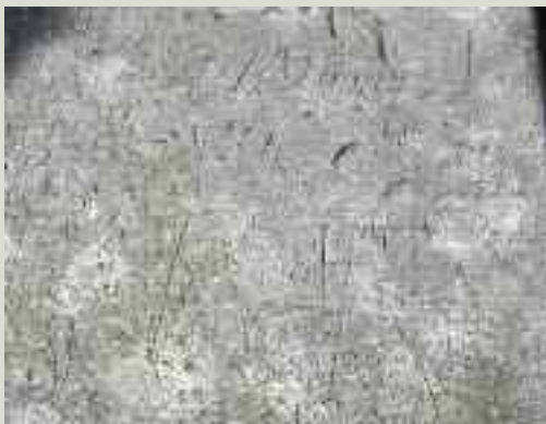
Lead sheet, while very durable, is soft. In this example, the lead sheeting has been etched with graffiti over centuries
