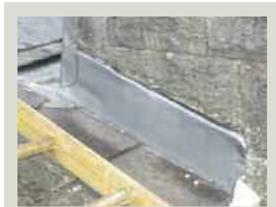
New lead flashing over lead soakers, turned into a mortar joint in the stonework at the base of a chimneystack and fixed using lead welts. The mortar joint is yet to be repointed
