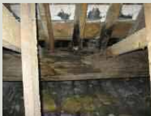
Evidence of wet rot damage to a roof beam and rafters under a tapered valley gutter. Only about ten per cent of the beam section was degraded, so no strengthening works were required to the beam. The rotted rafter ends, however, needed replacement
