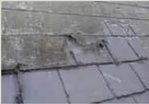
The process of covering a leaking slate roof with a bitumen covering was known as 'turnerising.' It is ineffectual and damaging and should never be carried out on a historic roof. Furthermore, it prevents the slates ever being salvaged for reuse
