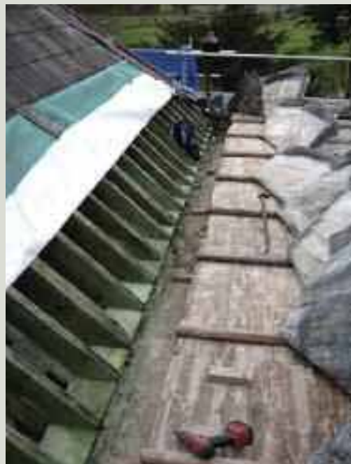
Slight lead corrosion can be seen on the exposed underside of the lifted lead sheeting on the right. The main problem here was a poorly detailed gutter. There was no need to change the regime of the flat roof, although good practice would include an underlay between the deal boards and the sheet lead
