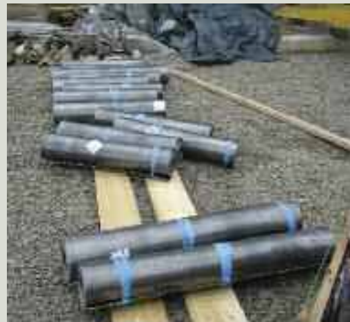
New lead sheet is supplied in rolls. Depending on the code specified, it can be exceedingly heavy and needs to be lifted with care. Despite this it is vulnerable to theft
