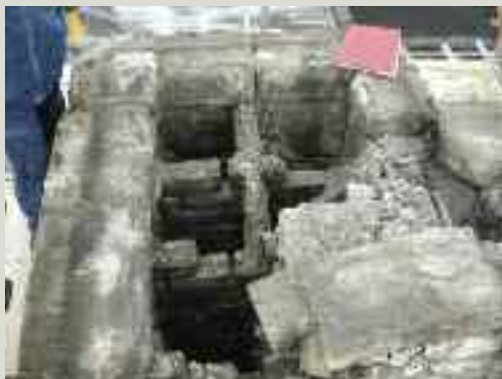
Many older flues have little more than half-brick fin walls called 'feathers' within the stack separating the flues from each other. These can be poorly tied in or even entirely missing as the result of chemical attack from soot, heat damage or over-vigorous cleaning with soot brushes
