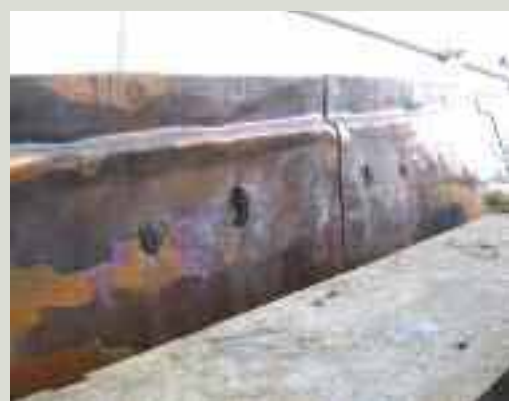
This copper parapet gutter lining has been lifted for inspection following water penetration problems. The bright salmon-coloured areas indicate that corrosion is occurring. Holes in the copper had been previously filled with a bitumen product in an earlier repair attempt which has exacerbated the problem, as bitumen corrodes copper
