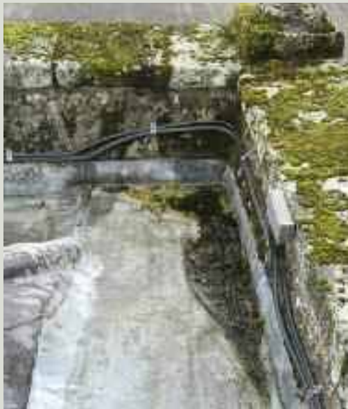
Ponding of water away from gutter outlets indicates a problem with the substrate timbers. In this case, a likely cause was poorly functioning flashings at the junction with the parapet wall
