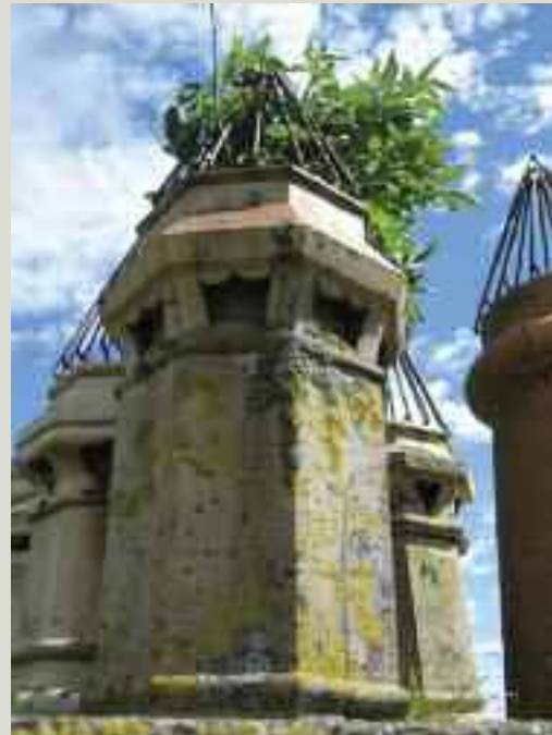
The use of wire crow guards prevents birds from nesting in chimney pots, but does not stop plants rooting in blocked flues
