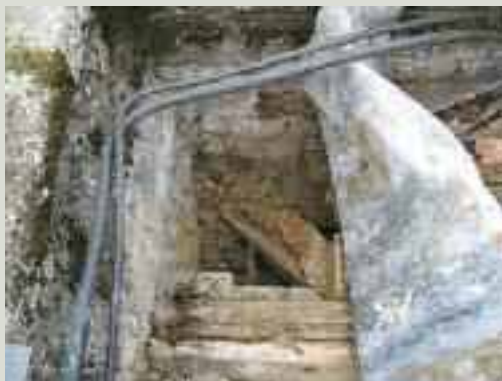
Rot beneath this section of parapet gutter resulted in localised ponding of rainwater, exacerbating the problem and leading to wet rot damage to the truss end. Note that bonding timbers embedded further down the wall may also be affected by such leaks
