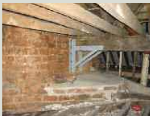
A new steel support bracket has been supplied to support this roof beam severely affected by wet rot at a chimney breast. The chimney flashings above, which had failed, were also repaired as part of these works
