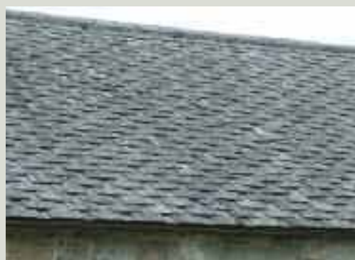
A method of slating sometimes referred to as 'open slating', 'hit-and-miss slating' or 'Scottish cant'. This slating pattern economised on the number of slates used and was primarily used for outbuildings. It is difficult to repair without face-fixing and the amount of exposure of slate surface can make the slates brittle for reuse
