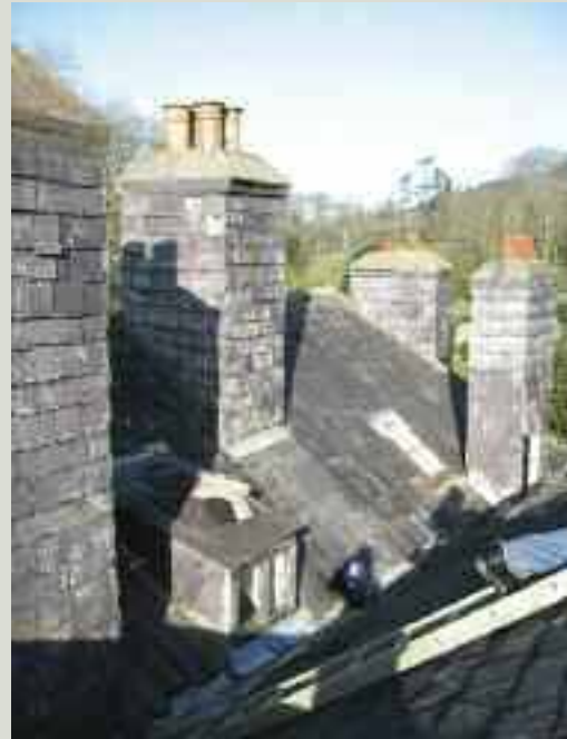
The change in colour of the slate on the chimneystack in the background indicates where a number of courses were removed and replaced. In areas of extreme weather exposure, vertically hung slating gives increased protection to the stacks
