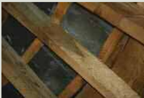
The use of a traditional scarf joint repair to damaged rafter ends is particularly worthwhile where the roof structure is exposed to view (Image courtesy of the Irish Georgian Society)
