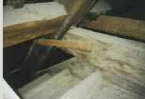
The extent of movement in this roof truss is serious, indicating not only the poor quality of the original detailing but also potentially serious movement in the main supporting walls below
