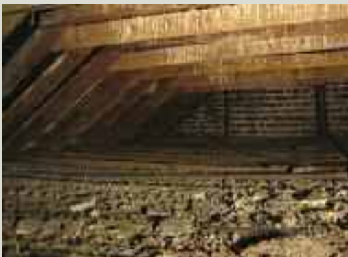
Undersized, long-spanning ceiling joists in this late eighteenth-century roof have become overloaded with pieces of fallen parging and pigeon guano, leading to deflection of the joists
