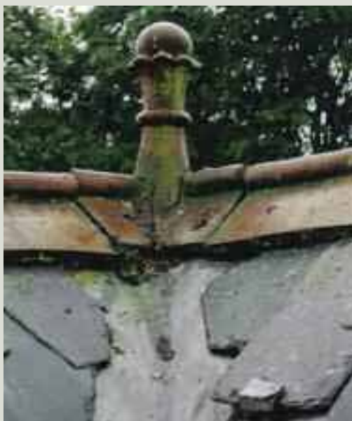
This terracotta ball finial was cracked; as part of a roof repair project it was removed, carefully cleaned and repaired before re-installment
