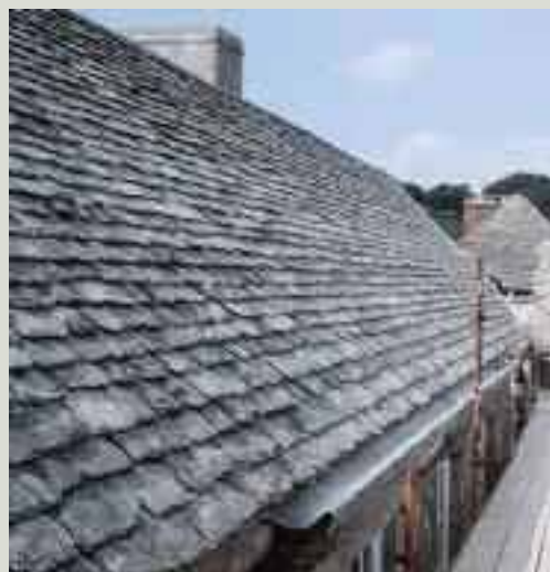
A new flush eaves gutter formed in lead along the top of the wall
