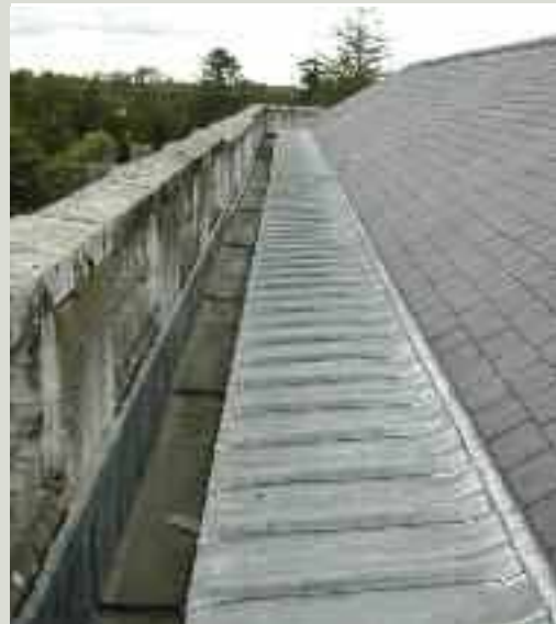
Welts to lead flashing to the vertical face of the parapet wall. Note the steps in the lead gutter and the rolls in the lead apron on the lower portion of the roof slope
