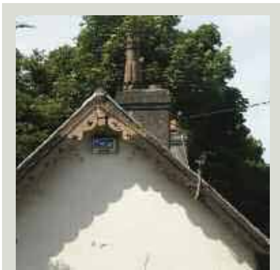
The poor condition of overhanging verges can lead to deterioration of the ends of the purlins as well as the loss of sections of decorative timber bargeboards
