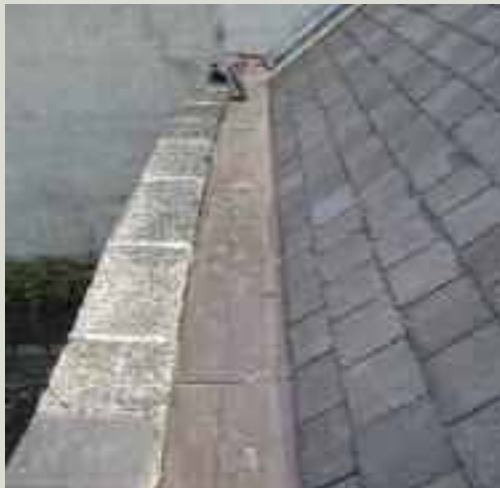
Parapet gutter re-lined in copper. The very shallow falls to this gutter precluded the use of lead
