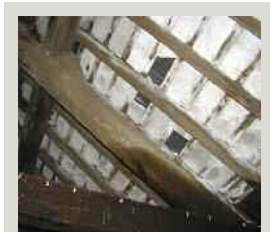
Substantially intact parging to the underside of slates is visible from within the attic space and provides a secondary line of defence against rain and wind entering the interior of the building
