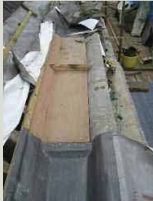
The design of this parapet gutter has been revised to achieve correct lead sheet lengths, falls and step heights in order to ensure that the newly-laid gutter will achieve a good lifespan. Note that the lead sheets have been fixed at the top end only (to allow for expansion and contraction), using copper nails in a staggered pattern
