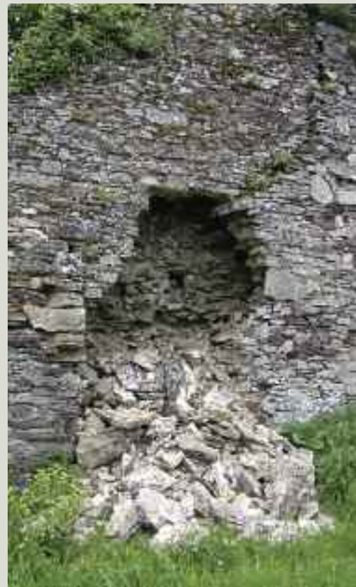
A partial collapse of the town wall of Youghal, County Cork. Recently-collapsed structures should not be approached until after a structural engineer has deemed it safe to do so
