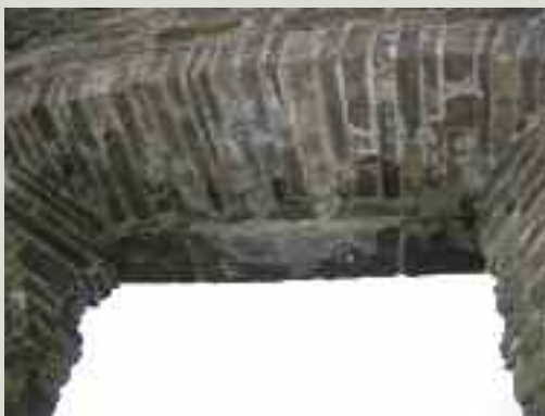
Failed lintel with stainless steel rods used to carry out a stitch repair
