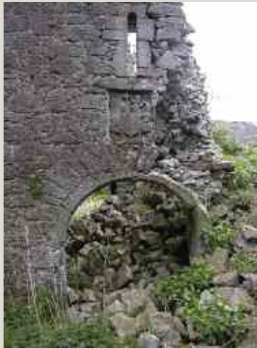
Partial collapse of this church tower occurred suddenly, taking down a portion of the nave wall
