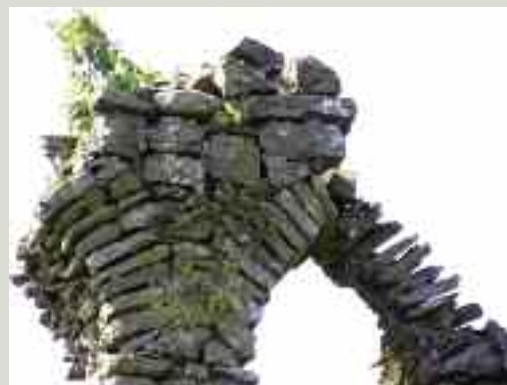
One arch on this double bell-cote has already failed. The other is on the point of collapse due to loss of mortar through erosion and exposure
