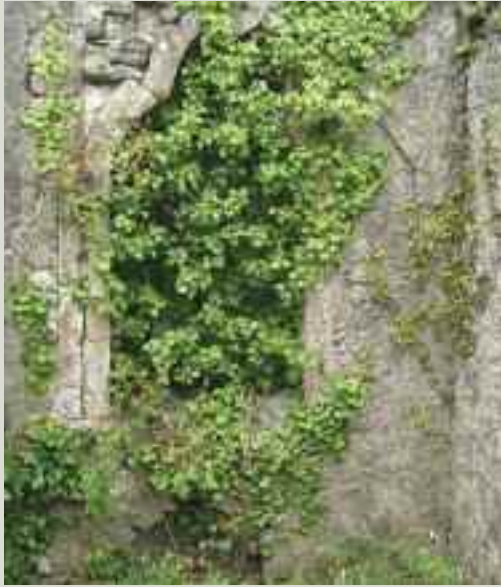
Ivy can become established within a masonry wall, growing unchecked through the joints and re-emerging in other parts of the structure
