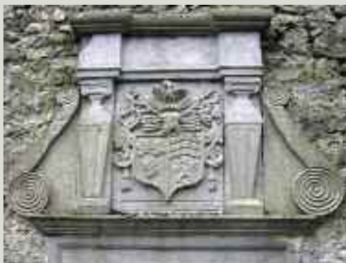
A ruin may contain fine carved features such as this tomb set into the wall. The condition of the carving should be monitored to ensure that no excessive weathering is taking place
