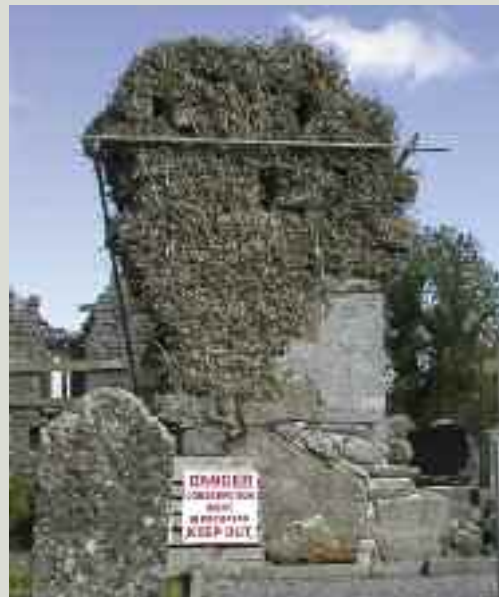
A clear sign warns of conservation works in progress. The temporary works to the wall in the background include scaffolding poles to provide restraint. The concrete blockwork on the right hand side provides temporary propping pending reinstatement of the wall core
