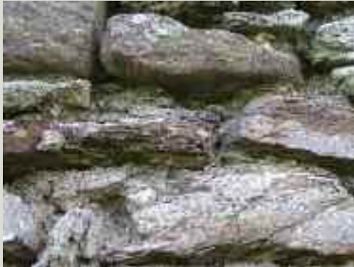
Decayed/weathered lime mortar
