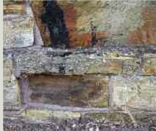
Delaminating stone, bedded vertically
