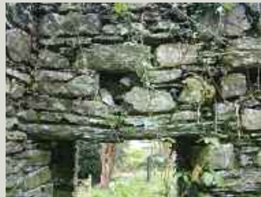
Lintel failure in this case was probably the result of the loss of mortar and stone from the wall above the lintel which damaged the natural self-arching tendency of the masonry placing excessive loading onto the lintel
