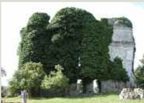
Vegetation which is allowed to grow unchecked can rapidly overwhelm a structure and accelerate its decay
