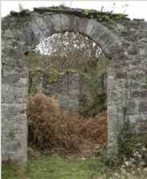
Arch over a door opening. This arch is also vulnerable because the wall over the arch has been lost
