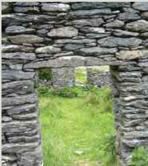
Stone lintel over a narrow opening. The thinness of the lintel, particularly at the right-hand end, makes it vulnerable to cracking
