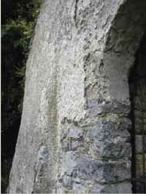
A wall showing surviving traces of external lime render. Most rubble-walled buildings were originally rendered to keep rainwater from penetrating into the interior
