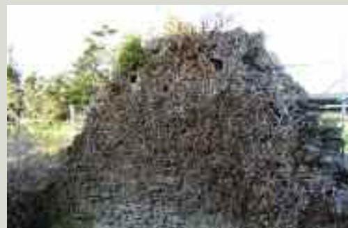
The top layer of vegetation has been sprayed and killed off pending its removal. The treatment allows for assessment and recording of the masonry
