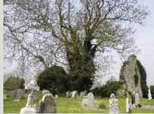
Mature trees adjacent to a ruin present a challenge. While they may add greatly to the beauty, character and natural heritage of a site, they can cause damage by undermining the foundations with their roots, or by falling branches
