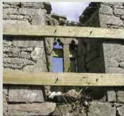
Timber bracing in the vertical plane to secure a window opening where a collapse outwards was imminent. The temporary work consisted of planks bolted through the opening
