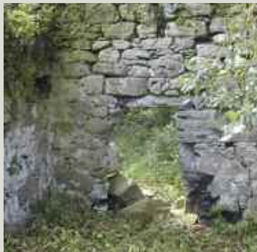
The stones that formed the jambs to this doorway have become dislodged because of cattle pushing through the narrow opening
