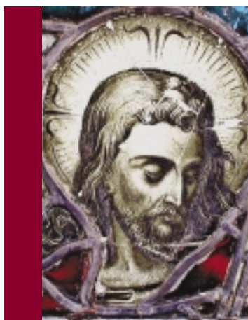
Detail to damage to window at St. Michael's Church, Ballina, Co. Mayo. Glass damaged in this way must not be replaced with a replica. It should either be left or repaired, thereby preserving the artist's original work.
